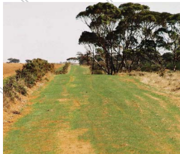
Land recovery after cable laying occurs quickly, leaving the land clean and more importantly, free of pylons.
